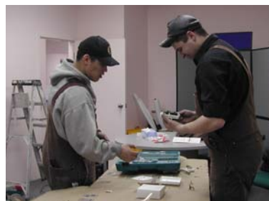
Bobby Makpah and Steve Fitzpatrick working on the electrical system for the office.
