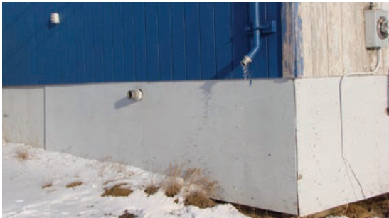
Skirting promotes permafrost thaw by warming the space under your house in the winter.
