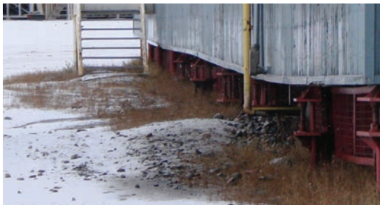
Uneven floors may indicate changing ground conditions.
