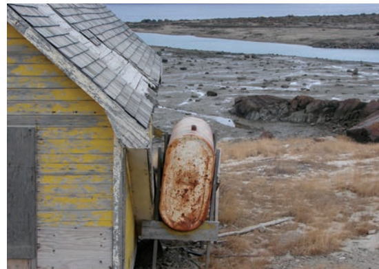
A wobbly or leaning tank can cause a break in your fuel line .
