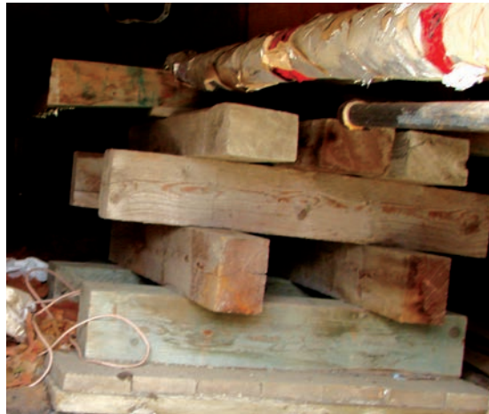
Permafrost degradation affecting foundations.
