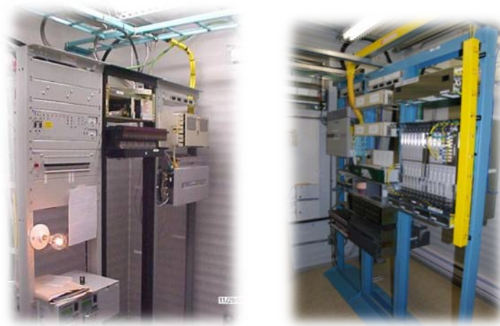
Figure 3 – Fibre Optic Terminal Equipment
