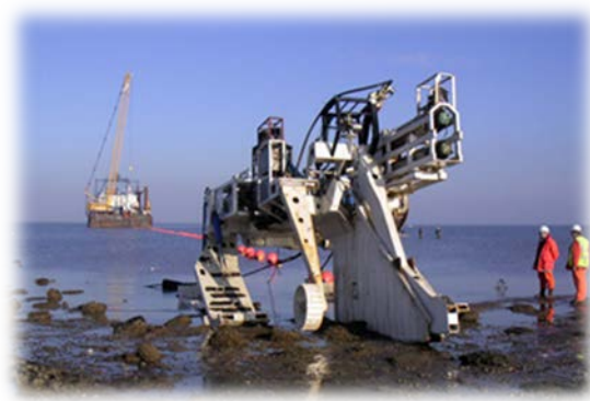
Figure 8 – Underwater Cable Plow
