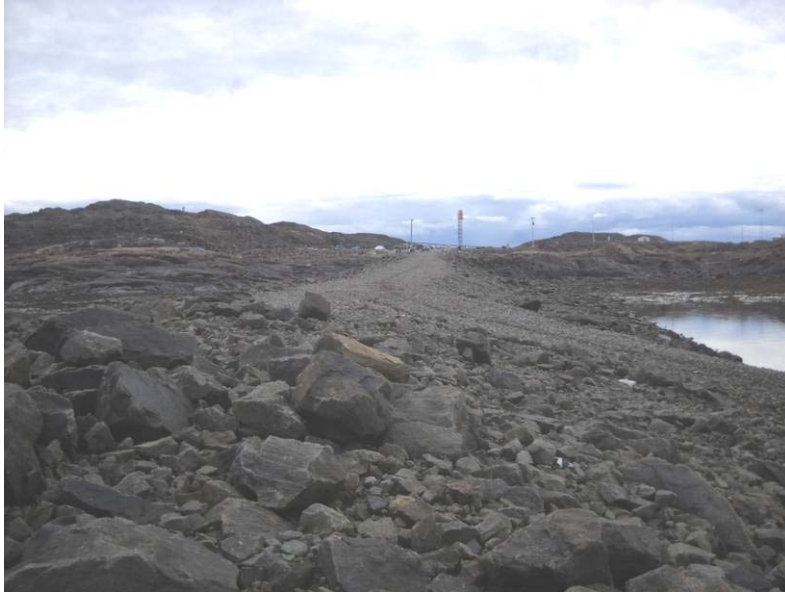
Figure K View from the bottom end of the Old Causeway toward shore. West side launching ramp is in the foreground. Tide at the time is estimated to be 2 m.
