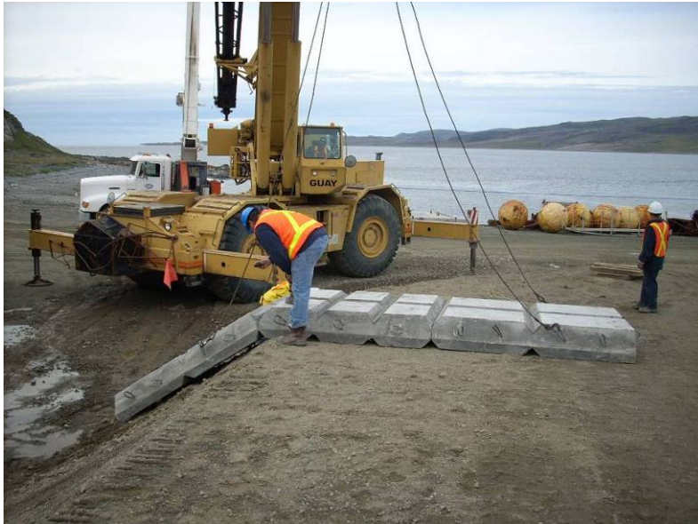
Figure R Scour protection mats.
