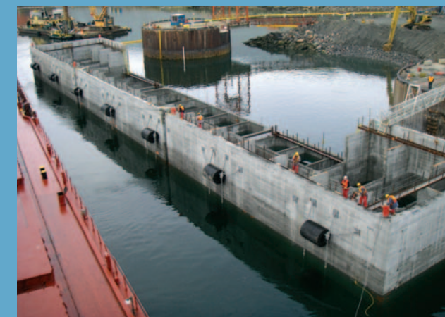
New Caisson Wharf Structure at Deception Bay Prior to Filling with Gravel
